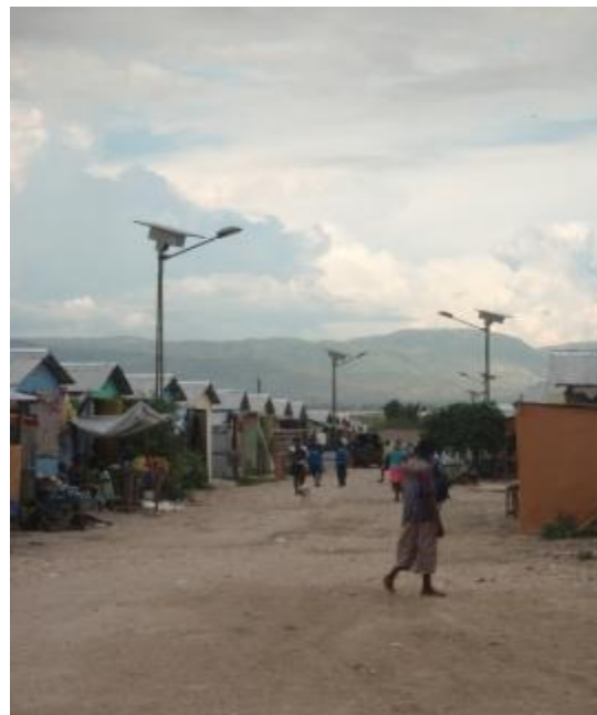
A view of the solar streetlights at the Caradeux Camp
